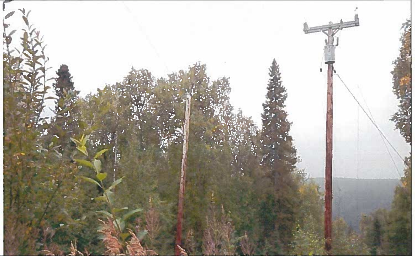
Overhead electric at Lot 8.
