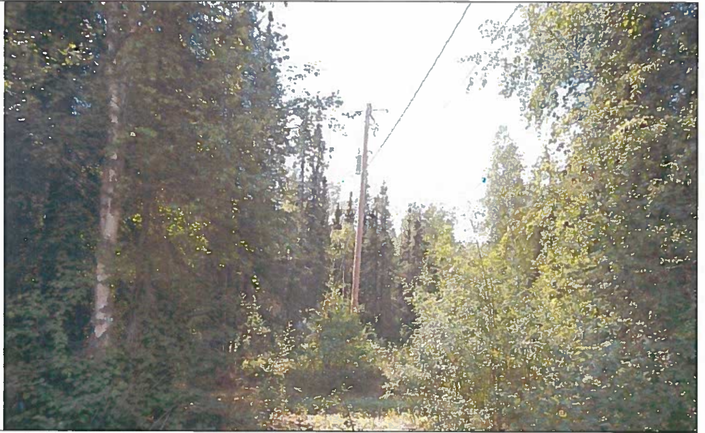
Overhead electric on the back lot lines of Lots 7, 8, and 9 in Block 4
