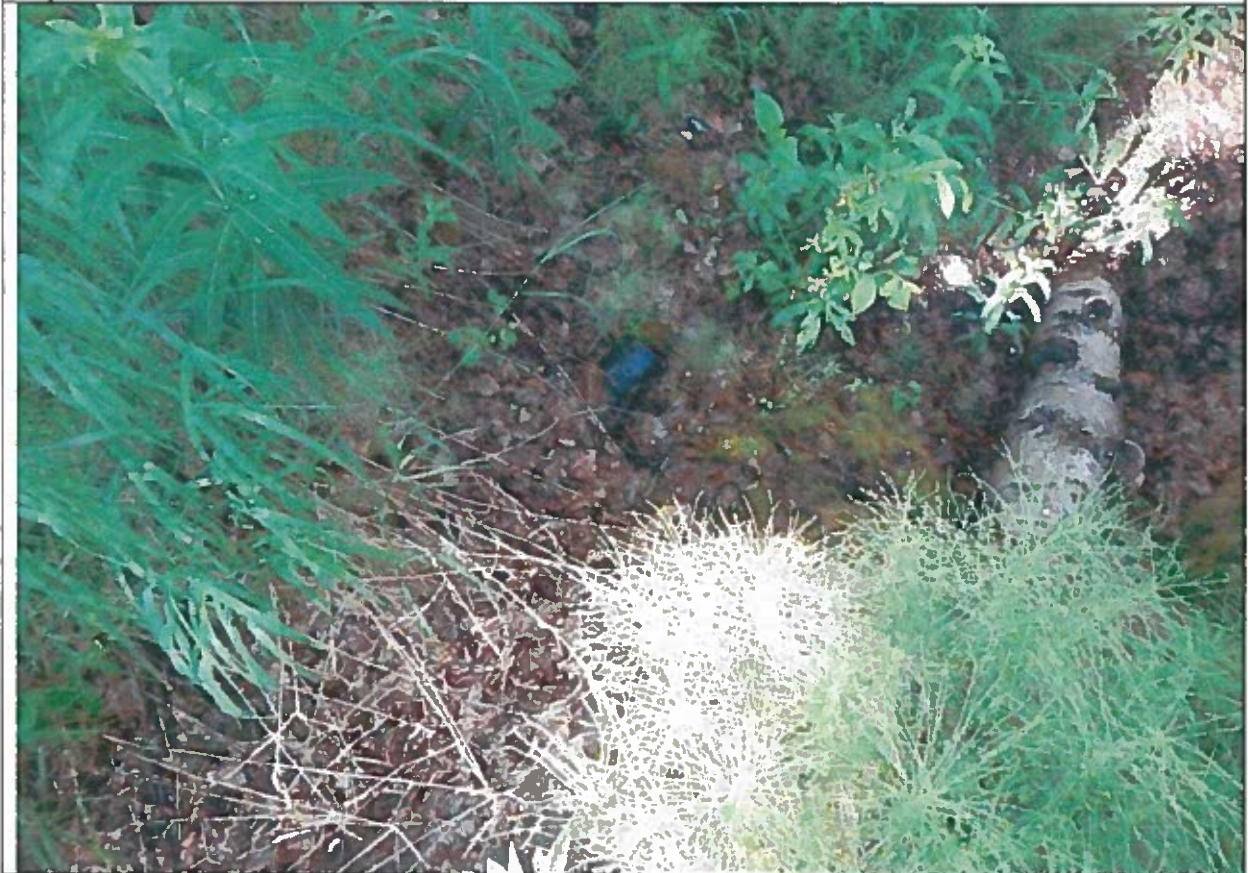
Vent pipe leads to hole prepped for septic. No system is in place.
