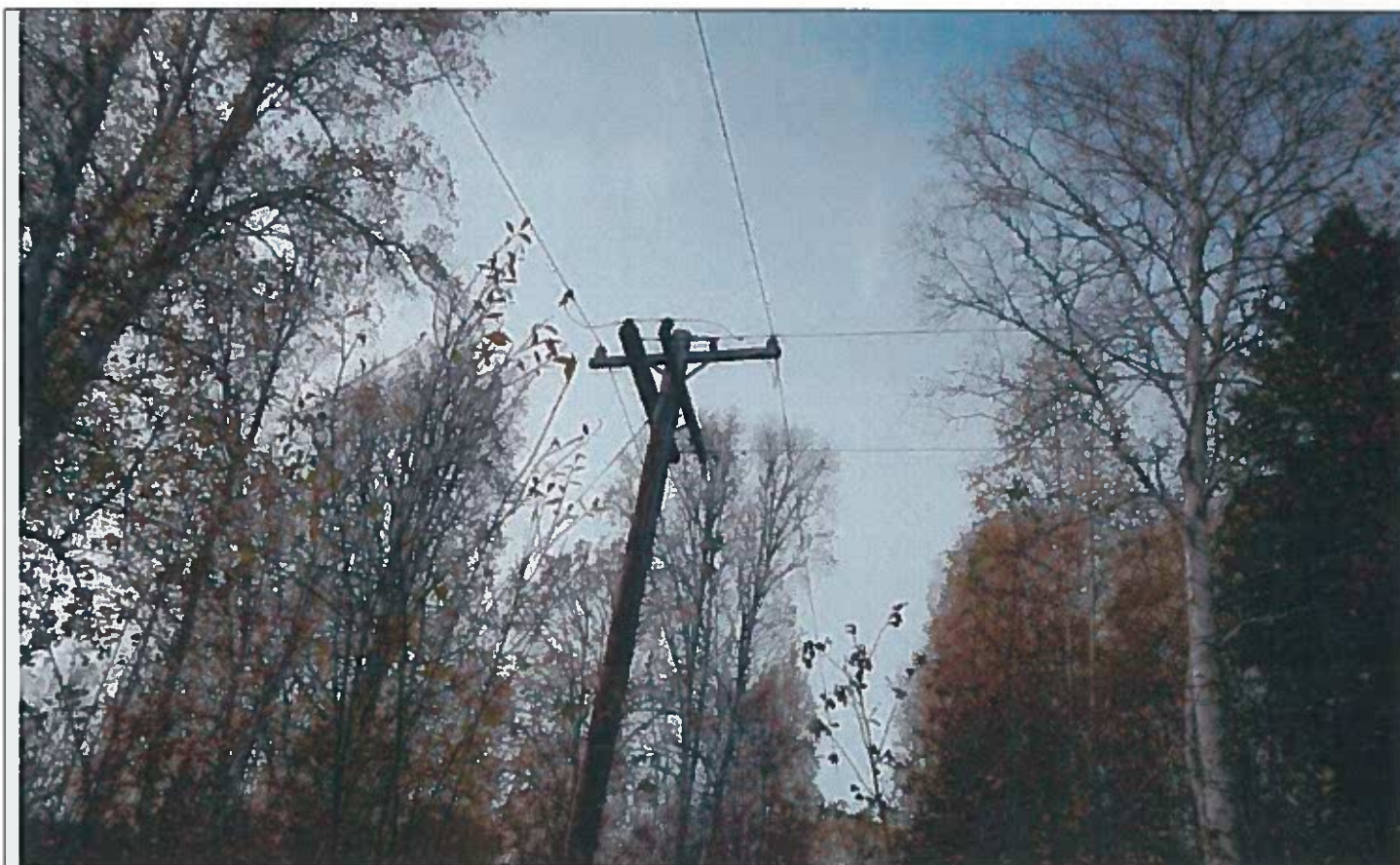
Overhead service lines in subdivision (MLW file photo) Existing lines on south side of subject lot line.
