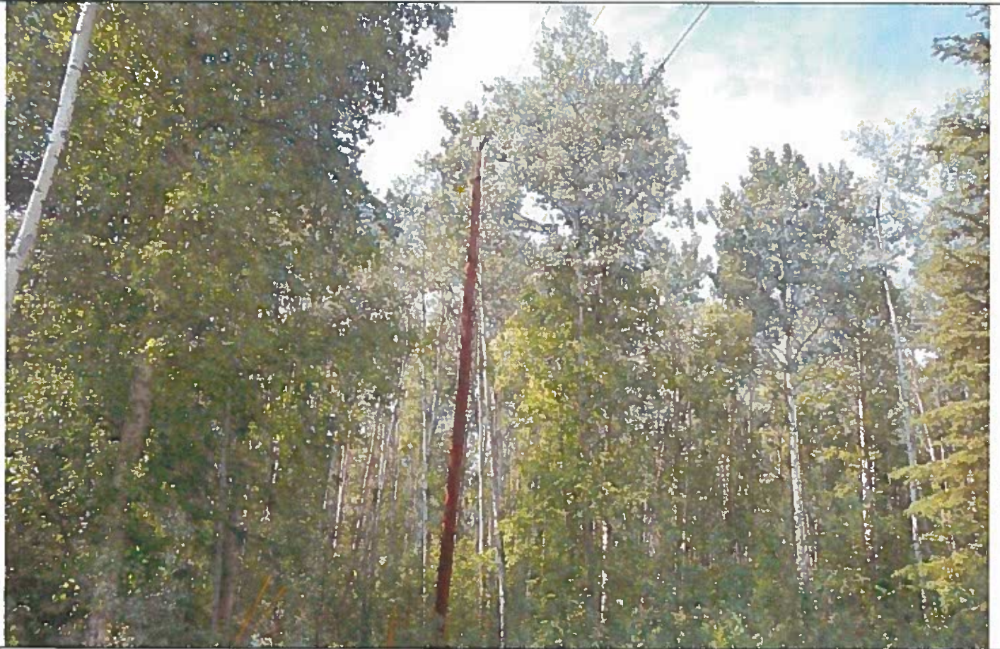
Overhead electric lines at the southwestern corner of Lot 7 Block 2
