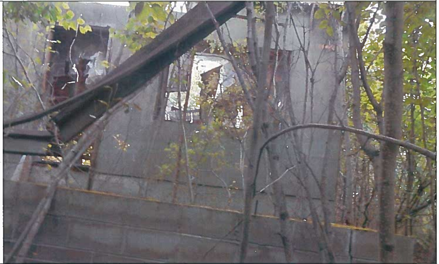
Dilapidated stick framing on block structure, no roof, doors, or windows.
