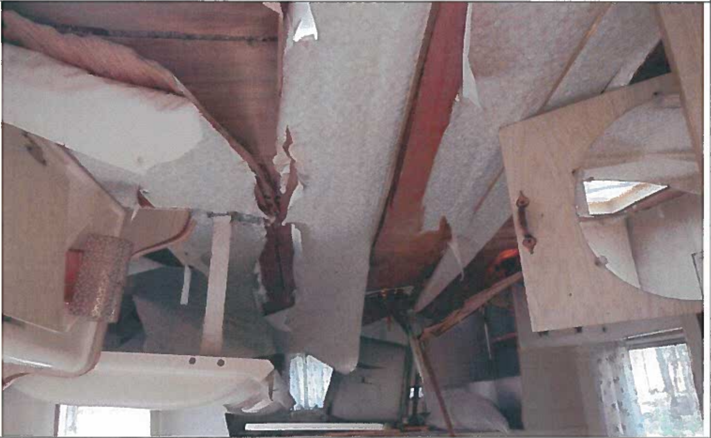
Cabover camper on ADL 418356. Roof caved in, open to the elements.
