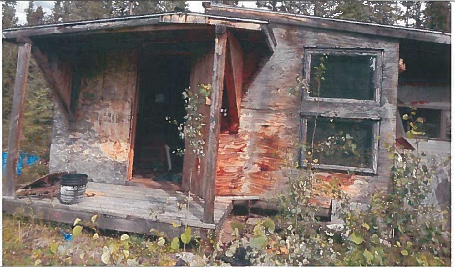
Dilapidated lean-to, open to the elements.
