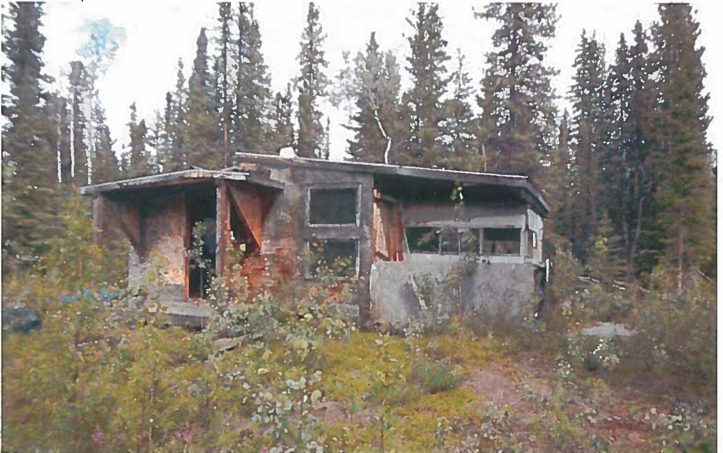
Dilapidated trailer and lean-to.
