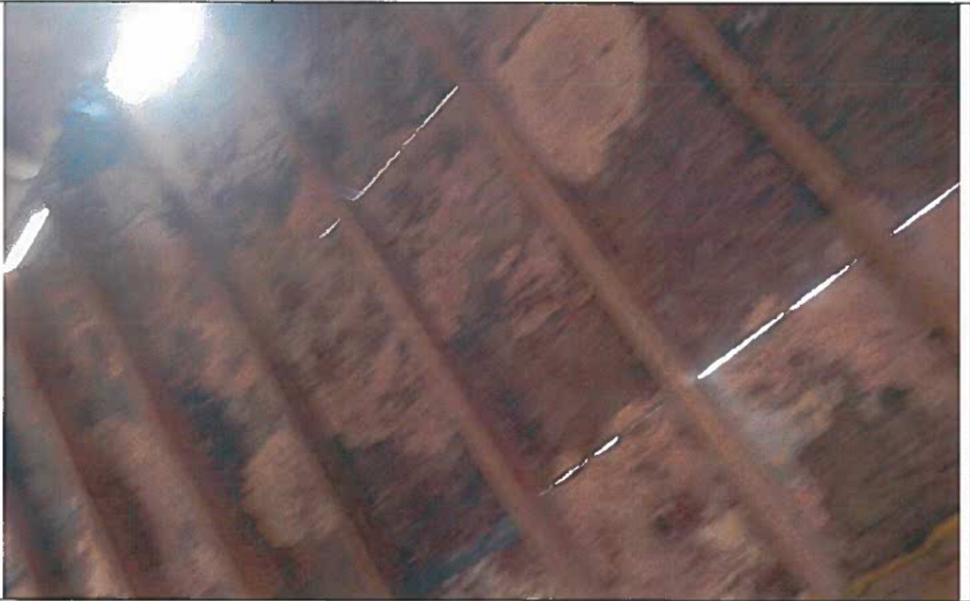
ADL 411192. Ceiling of cabin, damaged by weather.
