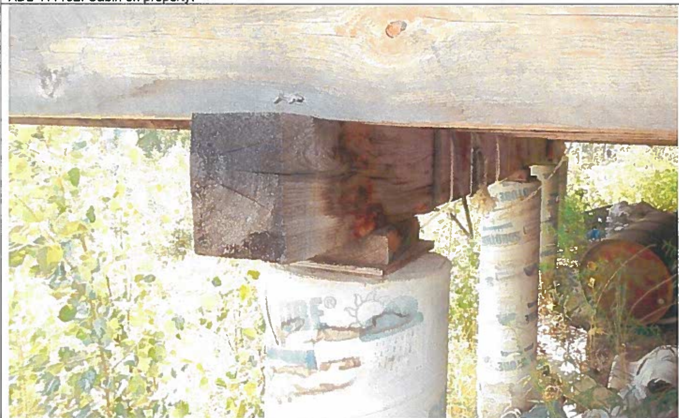
ADL 411192. Cabin foundation. Unsecured non-treated timber on Sonotube.
