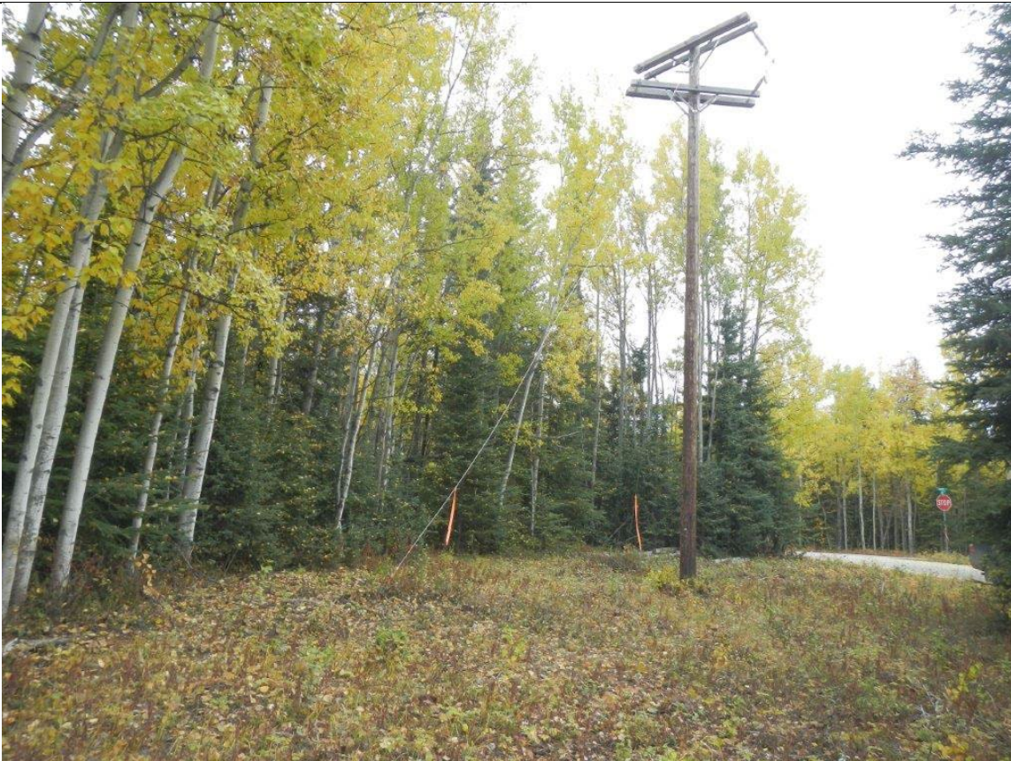
Lot 6 Block 2, Delta Townsite. Overhead electric.
