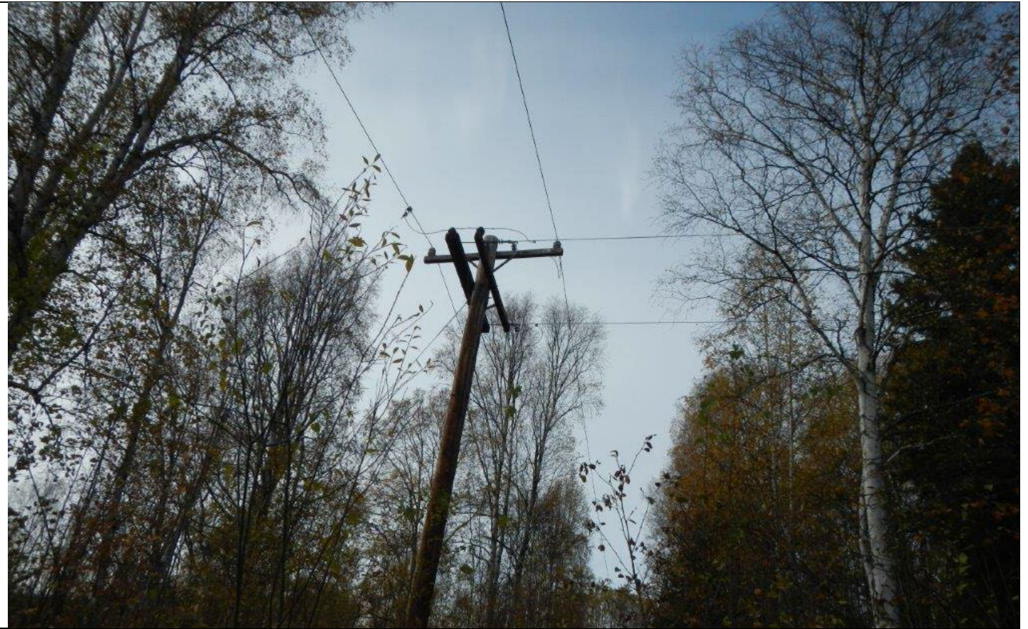
ADL 418603. Overhead electric near southeastern corner.
