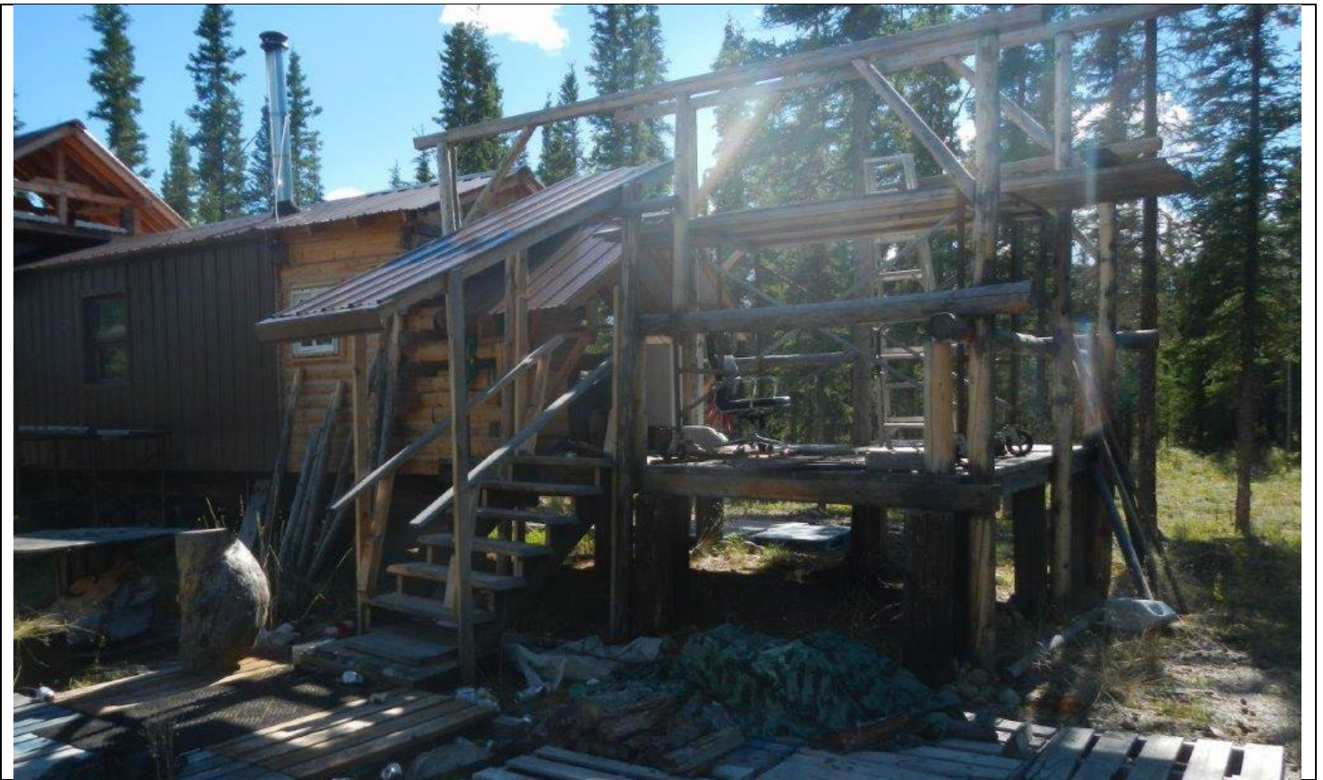
Porch built on pilings, abuts trailer and serves as landing. (MLW file photo)
