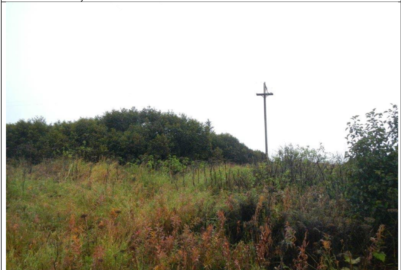
Overhead power on Lot 1 Block 1
