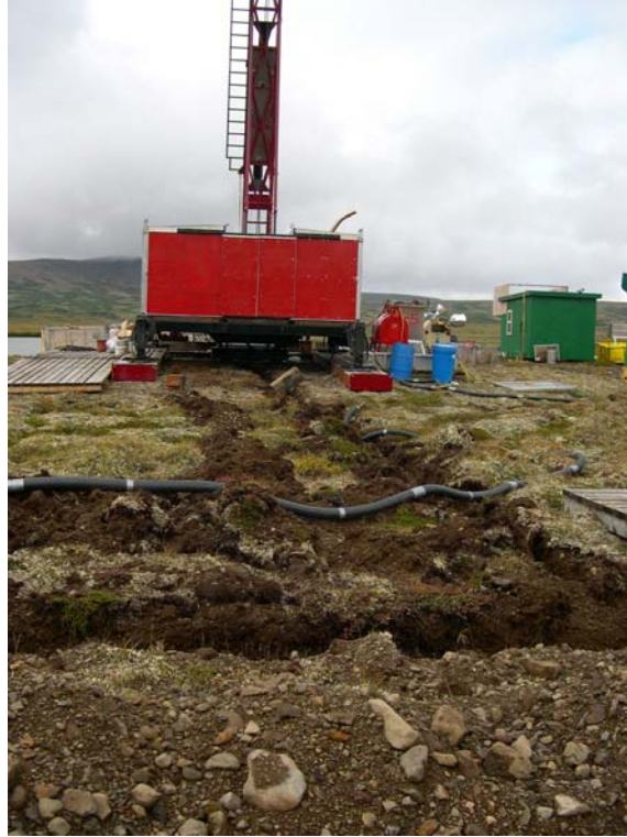
Figure 1. Rig no. 5 on new site. Trench leads from rig to sump pit.
