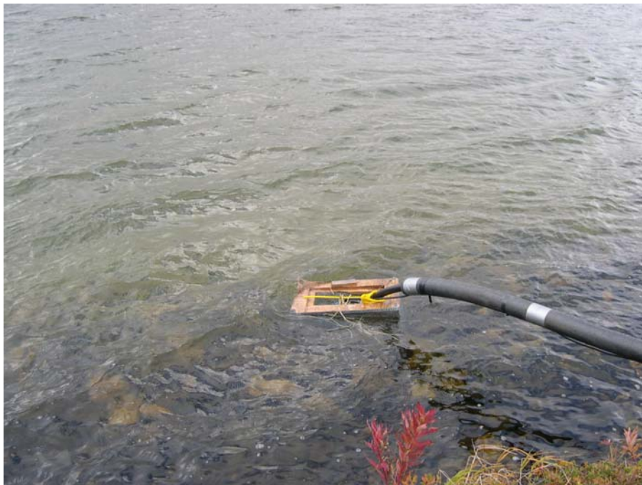
Figure 4. Water intake structure for drill site no. 7374 and for rig no. 5 new drill site. Note cover missing on intake box.
