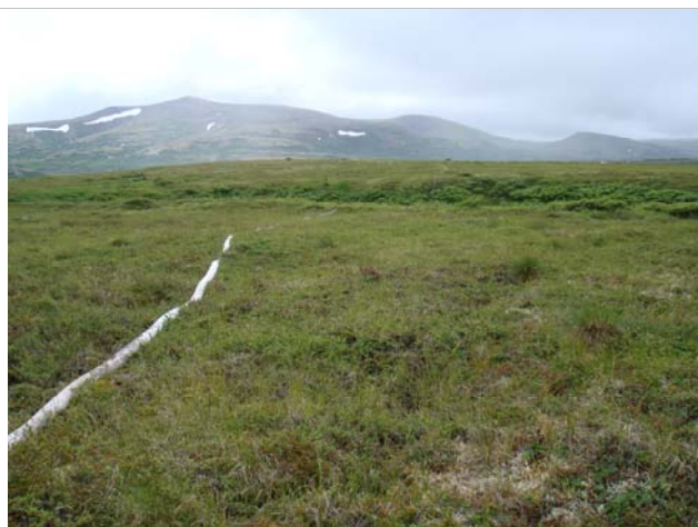
Figure 5. Drill discharge line from drill rig 2.
