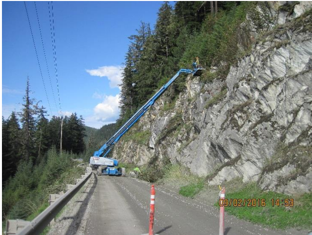
Photo 2. Contractors are brush cutting along the rock wall at the 1.9 mile B-road.
