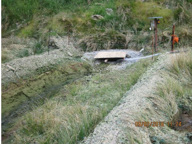
Photo 7. 1350 sump and caisson. The caisson and pump are protected by an electric fence.
