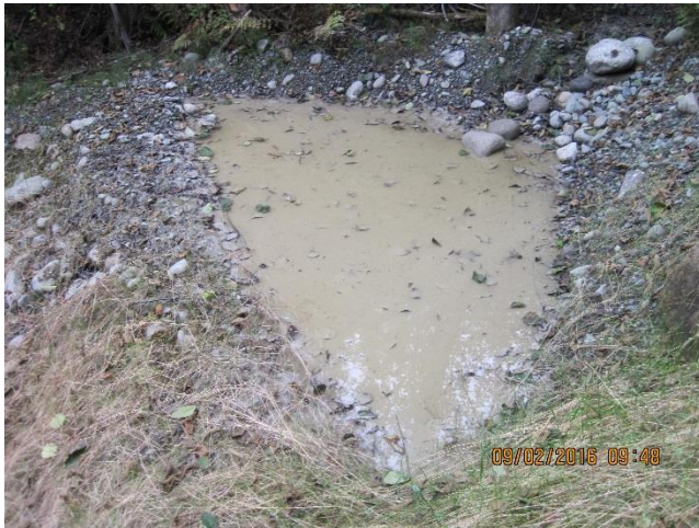
Photo 26. Zinc Creek Bridge uphill/downstream side sediment sump needs to be mucked.
