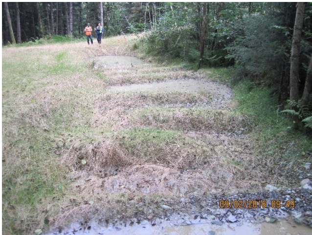
Photo 27. Zinc Creek Bridge uphill/downstream sumps and rock check dams.
