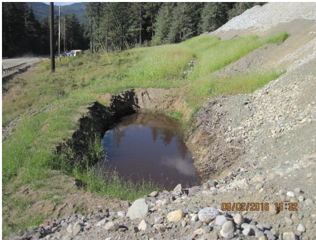
Photo 29. A sump for collecting stormwater runoff from the gravel stockpile at the 0.9 mile B-road.
