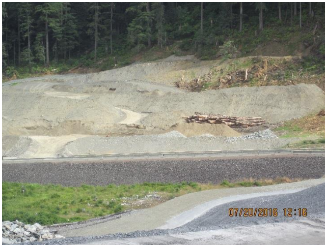
Photo 24. The stockpiled material at 0.9 Mile B-road area is for the TDF expansion project and for reclamation material.
