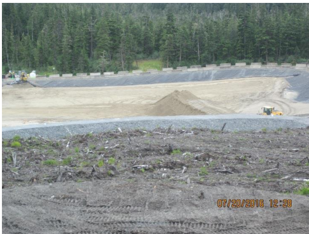
Photo 16. The liner for TDF expansion is installed and the service sand is being placed.
