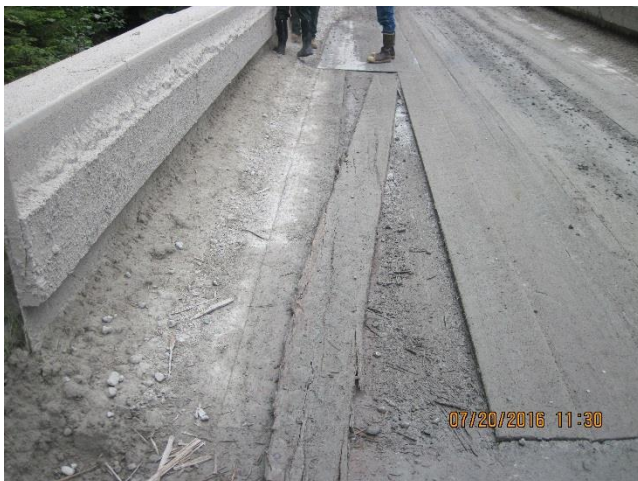
Photo 7. Falls Creek Bridge with two damaged wood planks.
