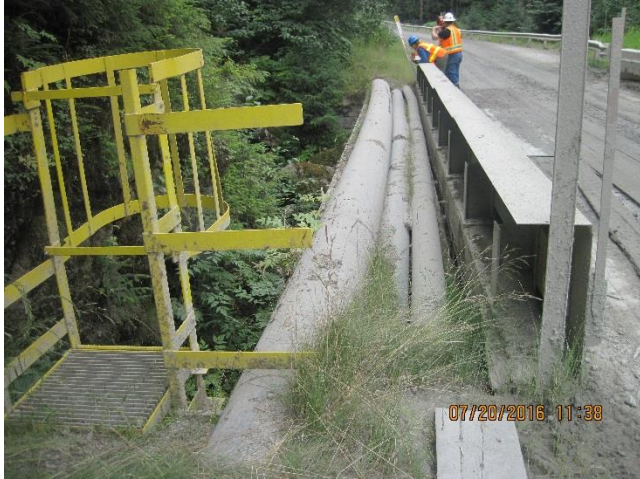
Photo 11. Sediment accumulating on pipes parallel to bridge.
