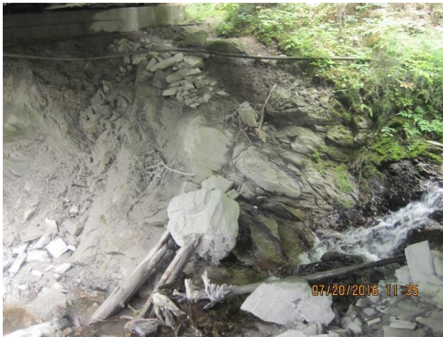
Photo 9. Sediments have accumulated on both sides of Falls Creek.
