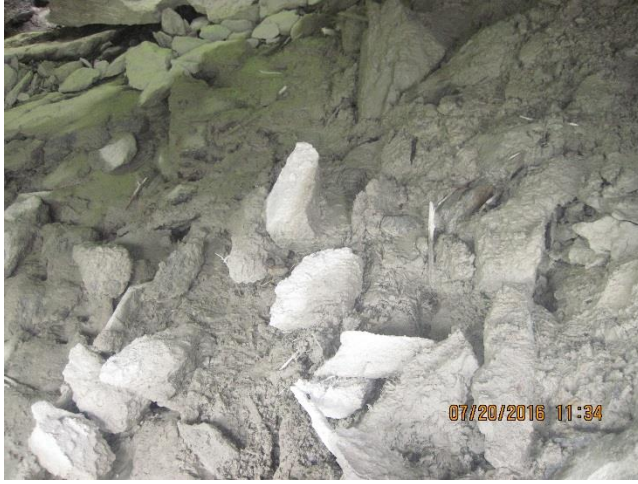
Photo 8. Sediments have accumulated underneath Falls Creek Bridge.
