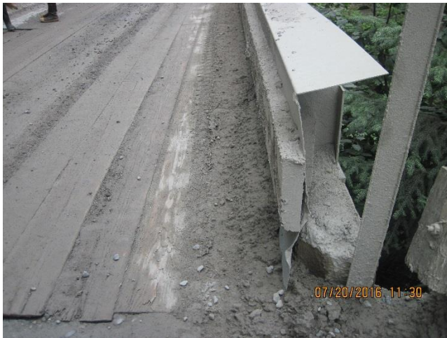
Photo 10. Sediment accumulating on the rails of the splashguards.
