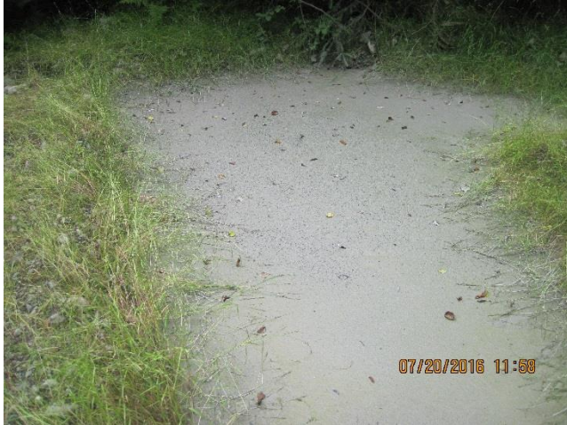
Photo 14. Sediment sump is almost at full capacity.
