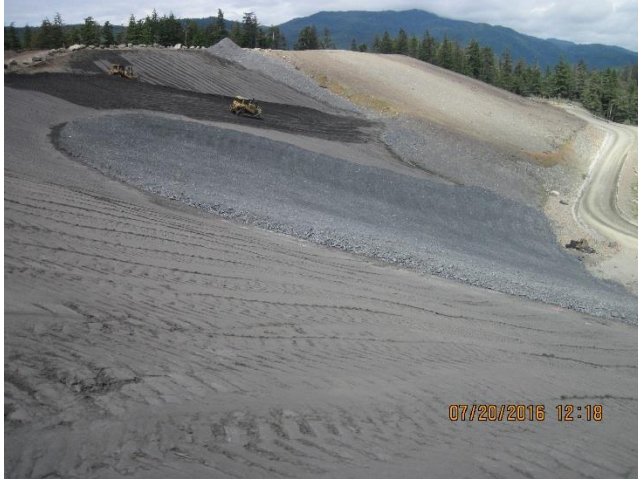
Photo 17. Class-1 waste rock (Argillite) used as armoring layer for the outer slopes of the TDF.
