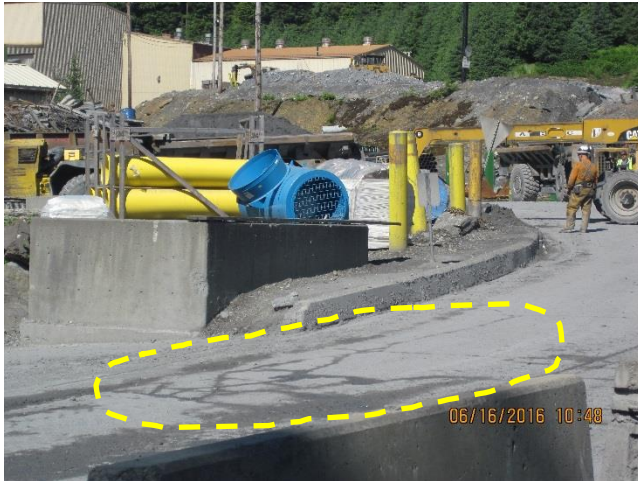
Photo 13. Dash line is the location of the broken 920 concrete overlay.
