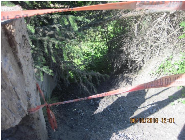
Photo 18. Sediments depositing below the edge of the bridge abutments.
