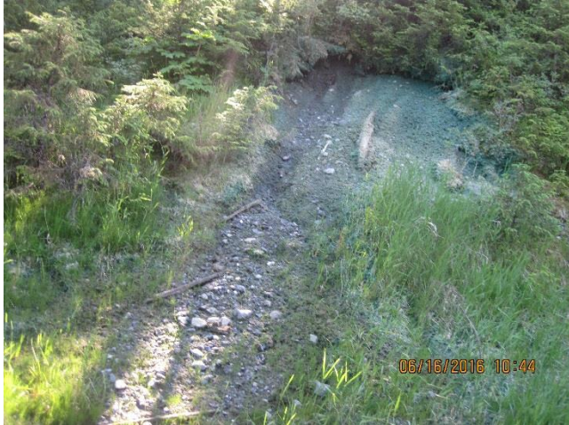
Photo 6. 1350 access road erosion along the hill slope.
