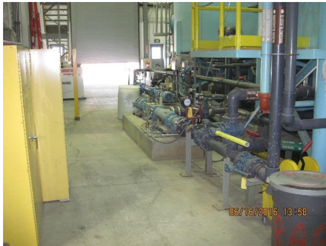
Photo 30. TDF water treatment plant.
