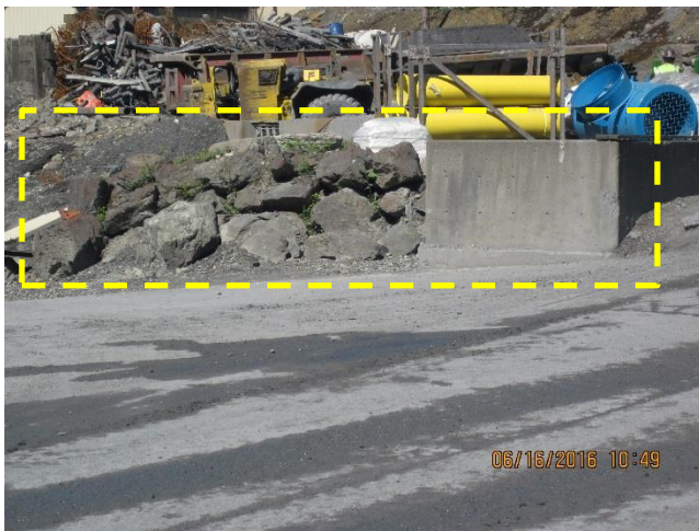
Photo 14. The rectangle is the location (920 area) that will be excavated in order reroute mine traffic.
