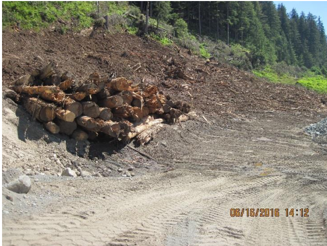
Photo 32. 0.9 mile B-road. The material stockpiled here is base material for the new lay down.
