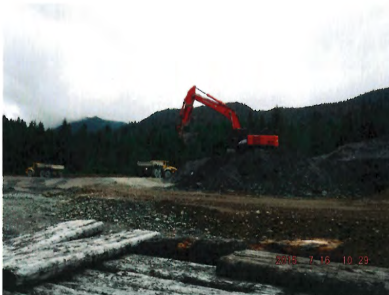
PHOTO 2. Waste rock removal from Site E (16 July 2015). Note the clean material placed for the haul road.
