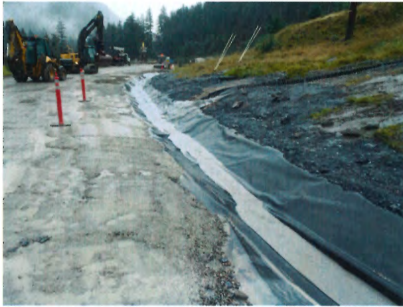
PHOTO 1. Lower section of reconstructed Site 23 Ditch and lower section of SmartDitch that conveys storm water off upper portions of Site 23 (September 2015).
