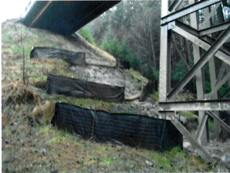
PHOTO 1. Northern bridge abutment BMPs (24 November 2014). The fencing seen in this photograph was designed to funnel sediment to a sump at the base of the slope and is operating as intended. A portion of the sump can be seen behind the base of the tower.
