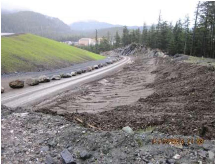
Photo 05. In October, till was placed to seal the west buttress quarry site at the tailings facility.
