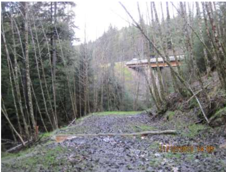
Photo 06. Stormwater runoff on the south side of Zinc Creek Bridge has been greatly reduced since our last visit in September.
