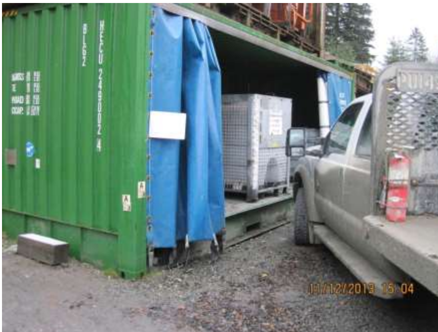
Photo 08. This sea van at the warehouse storage area at the mill has built in secondary containment. It stores vehicle fluids including antifreeze, transmission fluid, diesel exhaust fluid, and drivetrain oil.
