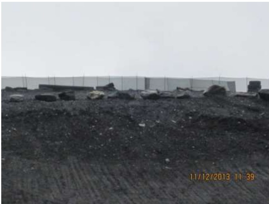
Photo 04. This snow fence is installed on the crest of the tailings pile during the winter months to reduce dust loss.
