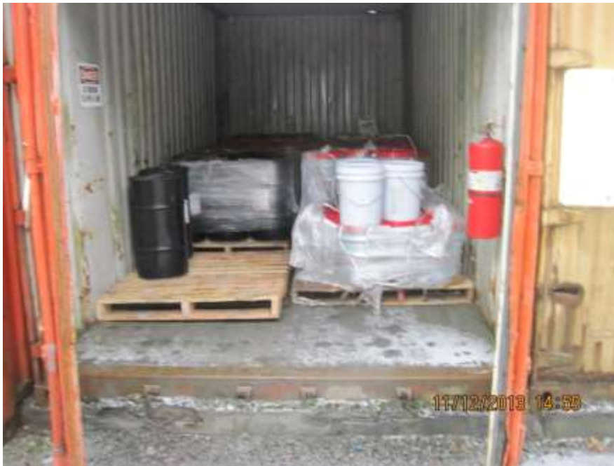
Photo 07. This sea van at the warehouse storage area at the mill is storing petroleum products (grease) without secondary containment. Also, the sea van is not on a concrete surface that drains to Pond A.
