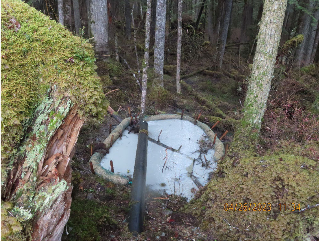
Photo 19. Turbid water was observed breaching the BMP straw wattle.
