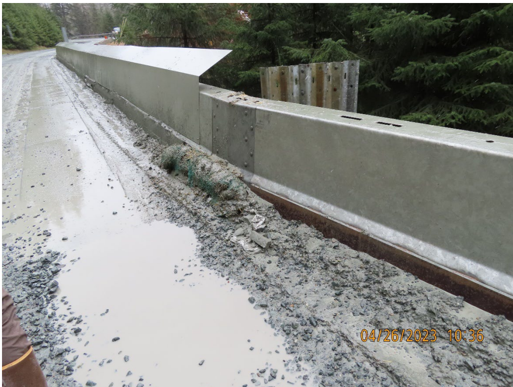
Photo 12. The downhill side of the 7.4 Bridge end requires sediment removal.
