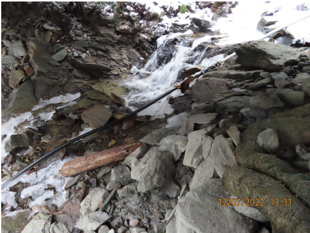
Photo 13. Area where turbid waters were observed entering Falls Creek from bridge abutment during previous inspection. Turbid water was not observed during this inspection.
