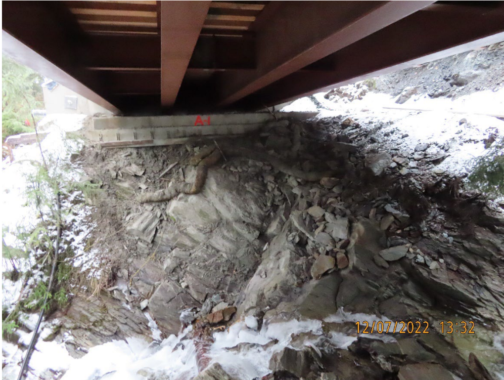
Photo 12. Falls Creek Bridge downhill side abutment BMPs in disrepair.
