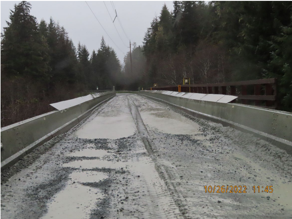
Photo 23. Zinc Creek Bridge with minor ponding of water.
