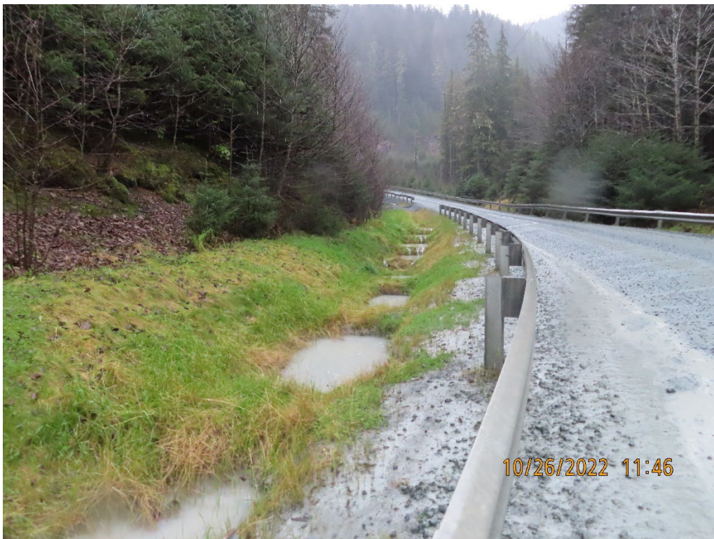
Photo 27. Small sumps above the Gnome Ponds that require sediment removal.
