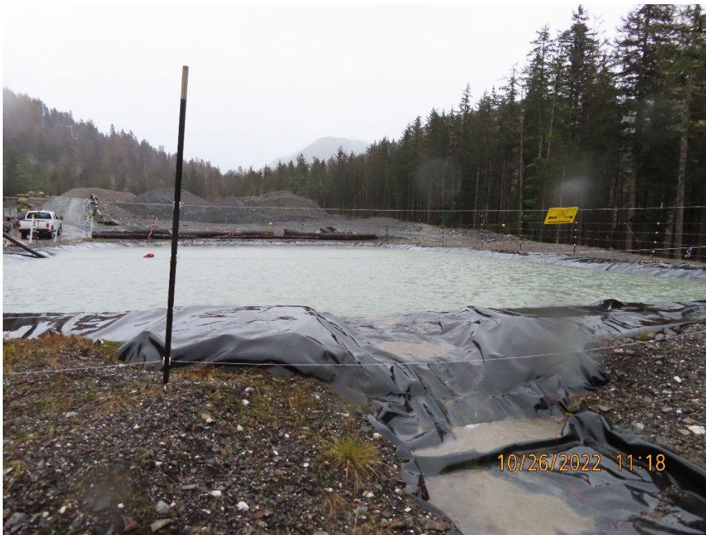
Photo 17. Stormwater pond at capacity at Site E.
