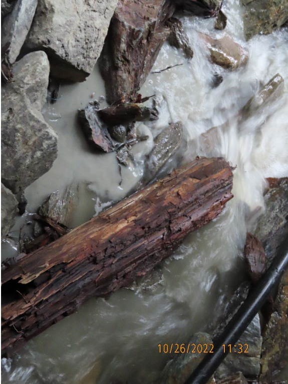
Photo 22. Turbid waters entering Falls Creek from bridge abutment.
