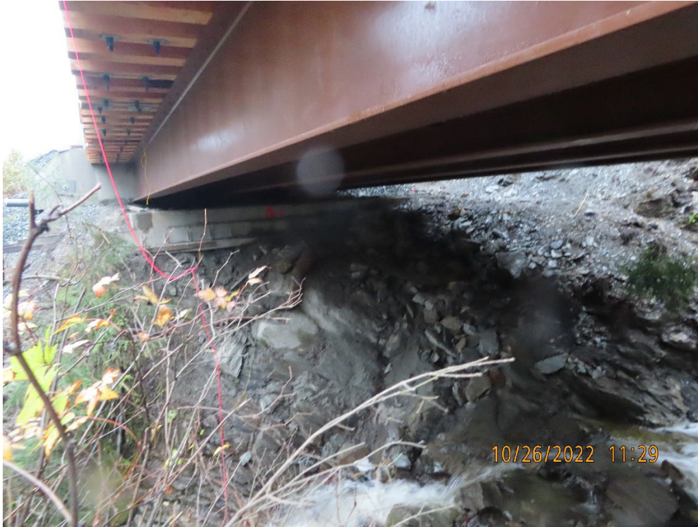
Photo 20. Falls Creek Bridge downhill side abutment BMPs in disrepair.
