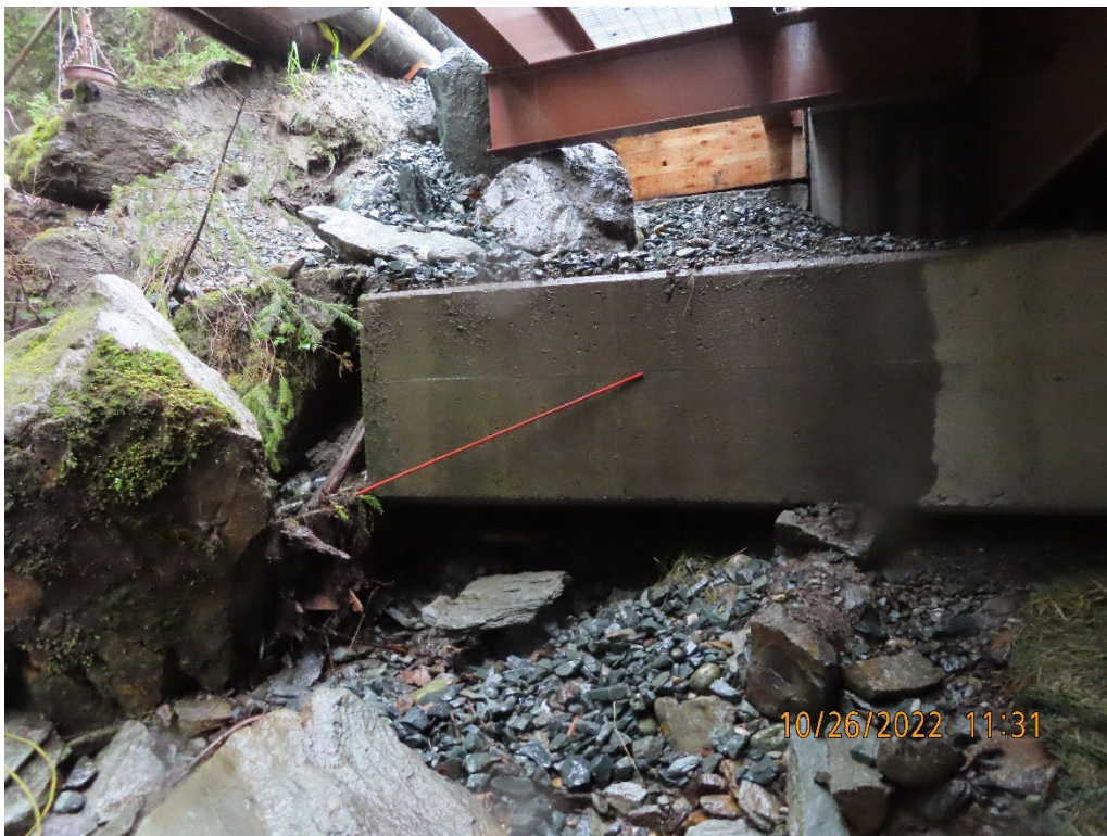
Photo 21. Falls Creek Bridge uphill side abutment BMPs in disrepair and likely source of turbid water.
