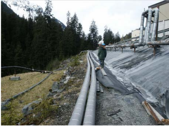
The dewatering pipeline that broke.
