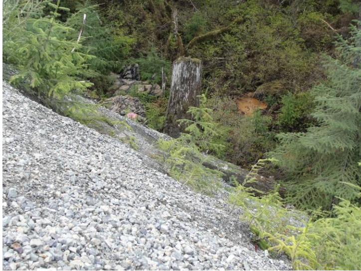
Mile 1.8 Pullout – Note Seepage at Toe of Slope
