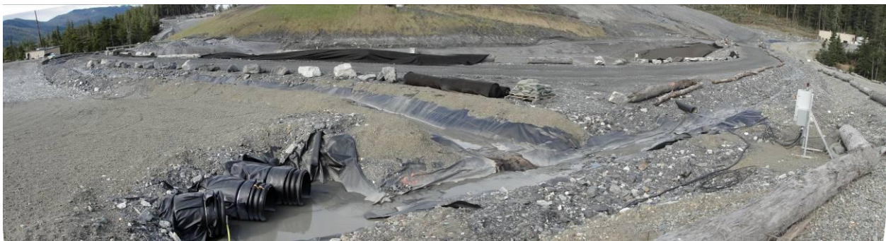
Southwest Tailings Facility Near Water Treatment Plant Showing Stormwater Collection and Controls
