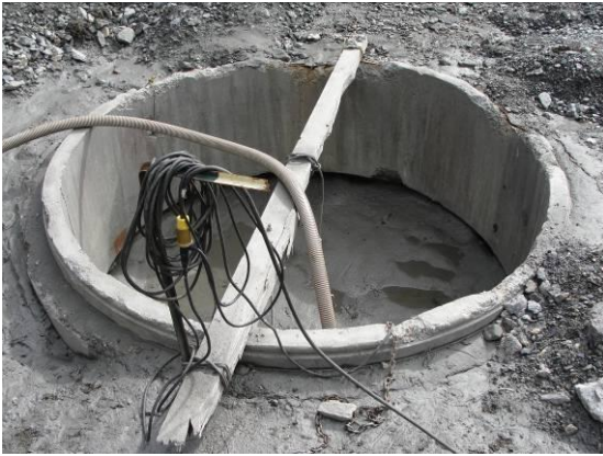
Sump at Site E
