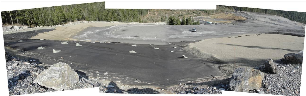
Tailings Disposal in the Northwest Pit 5 Area – Note: Sand Layer and Geotextile
