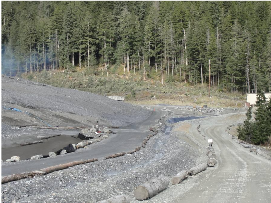
East Ridge Expansion at Tailings (Background) Stormwater Controls at South Tailings (Foreground)
