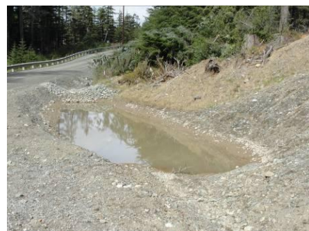
Settling Pond and Check Dam for Sediment Control
