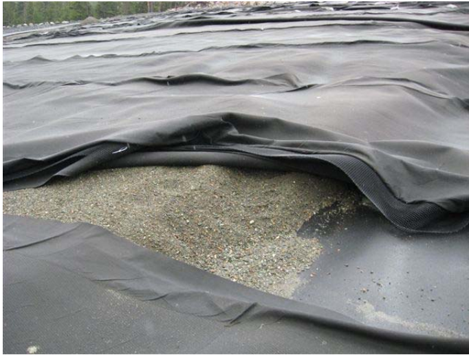
Geomembrane, geotextile and lower protective granular layer at the tailings NW expansion site.
