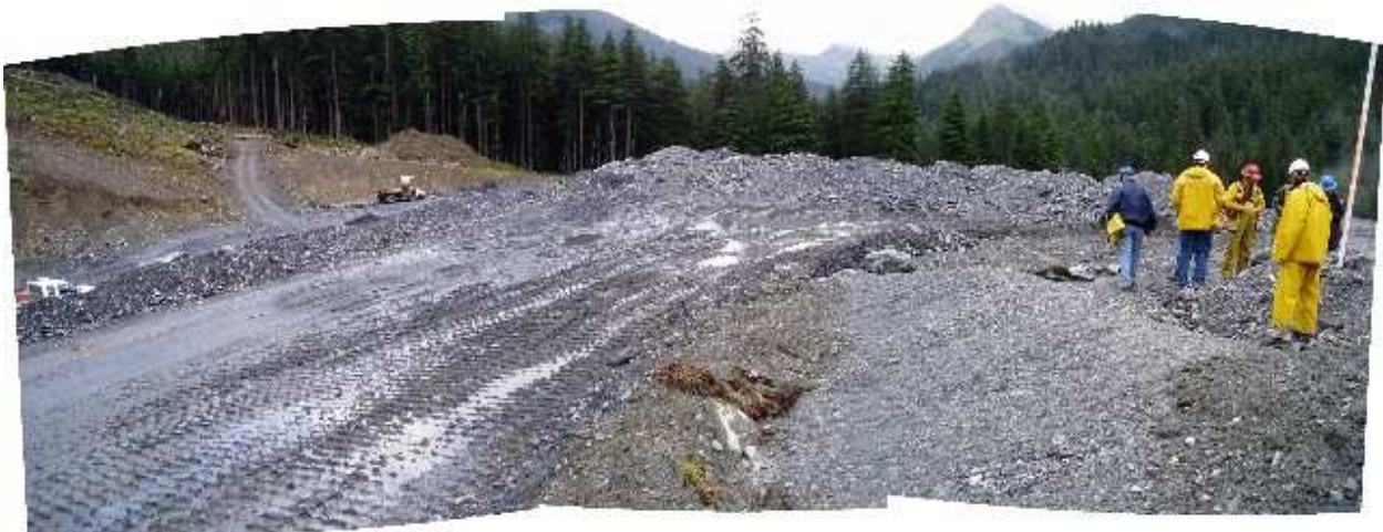
Differentiation of Class II and Class III waste rock placement zones at Site 23
