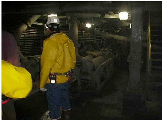
Paste backfill pump underground
