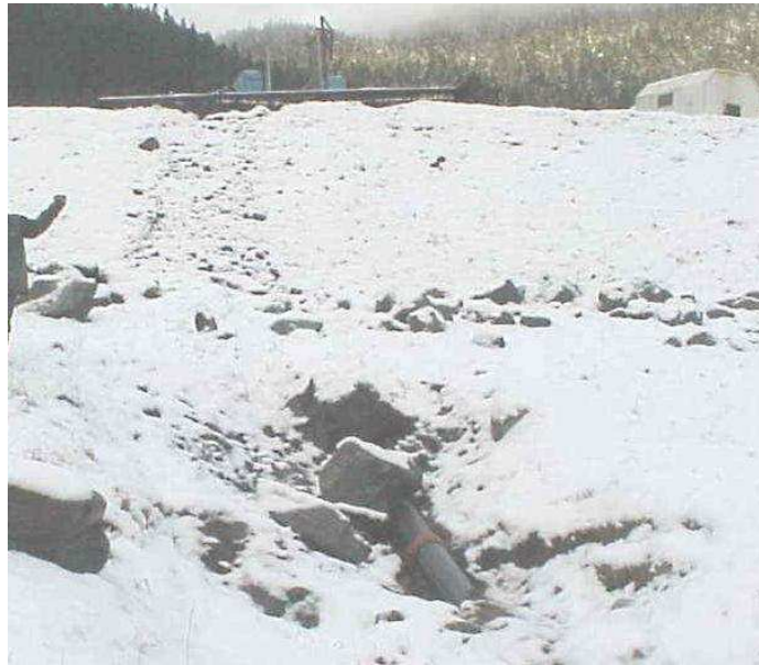
Drainage Pipe From Curtain Drain At Site D
