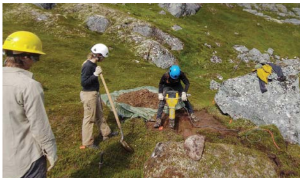
Trail crew on the Reed Lakes Trail in the Hatcher Pass Management Area
